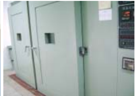
Temperature cycling test chamber
